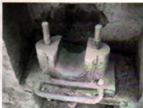
A pair of original 19 th century bolts which once held a machine in place.
